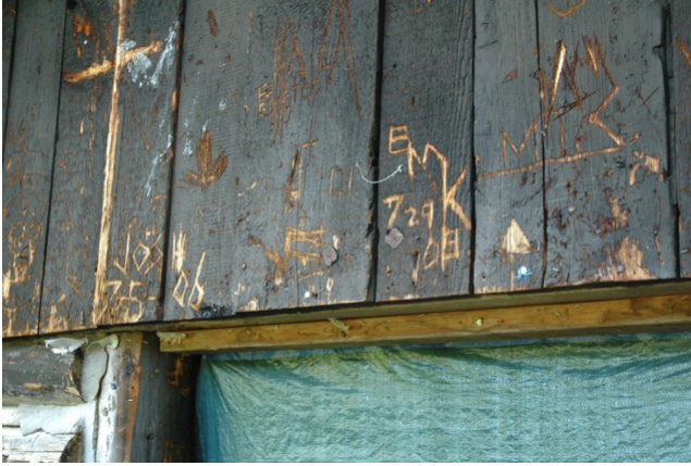
Graffiti on the river cabin in Green Timbers. Structure is unsound, DNR says.
