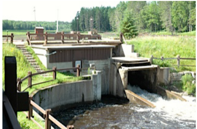
Dam across Pigeon to be removed late next summer or early fall and replaced by a bridge, if funds can be raised.
