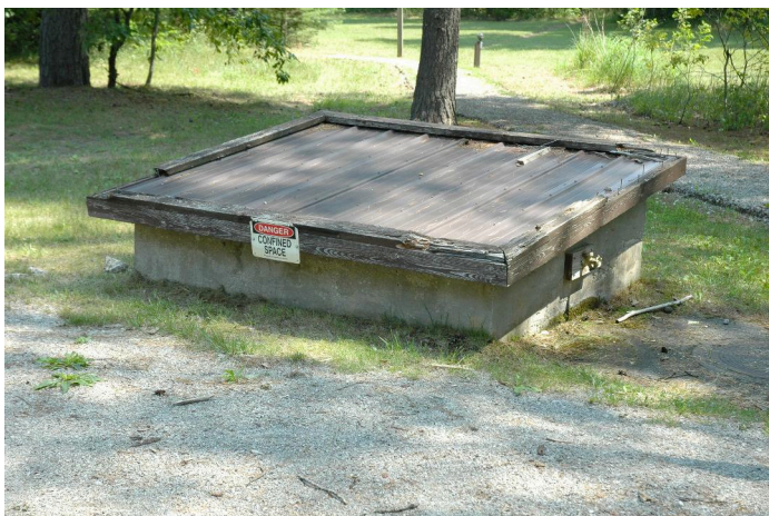
Replacing this 1932 water well is one of many items on the agenda for the forest's new unit manager, Mark Monroe.
