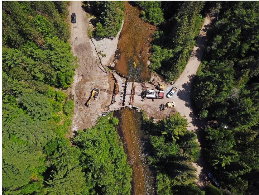
Washed-out east end of Ford Lake Road got a makeover as tubes in the Pigeon (flowing bottom-to-top in this view) were being replaced by a timber bridge. Photo by Dutch Neubecker
