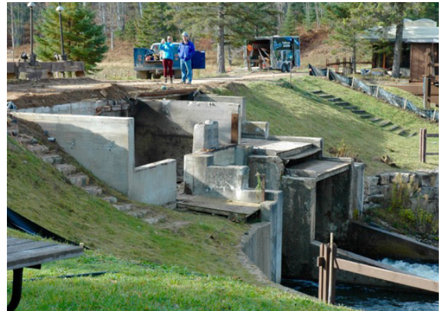
Lisha Ramsdell stands with Jeff Allen, job foreman, on ground just before his crew began removing it from the river along with just about everything visible between the two fences on the right.
