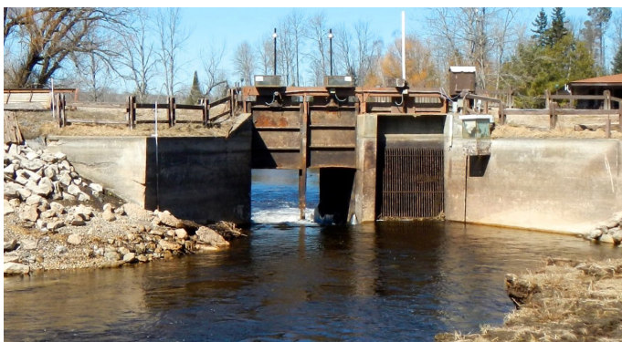
Dam still sits astride Pigeon River. As viewed from ground that used to be under the pond, the river flows into the open dam and on downstream beyond the opening. All structure is to be removed, except the dining hall on far right beyond the fence. | © Joe Jarecki
