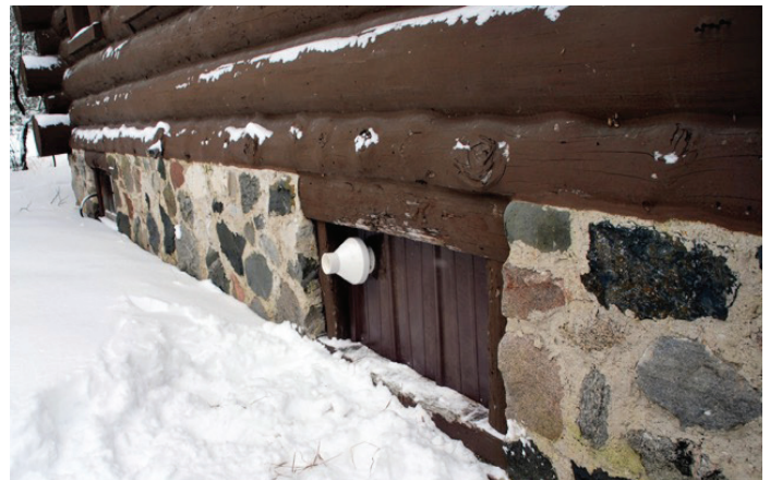
New propane heating system pokes a modest exhaust pipe out of the foundation as preparations continue for a late summer opening. © Rudi Edel
