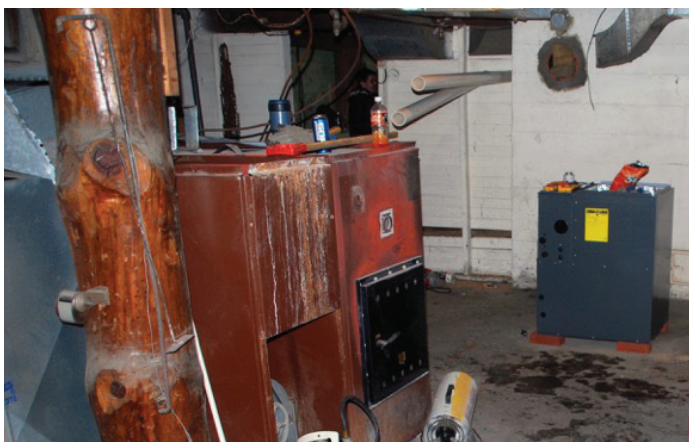
Old furnace sits next to log pillar in basement.
