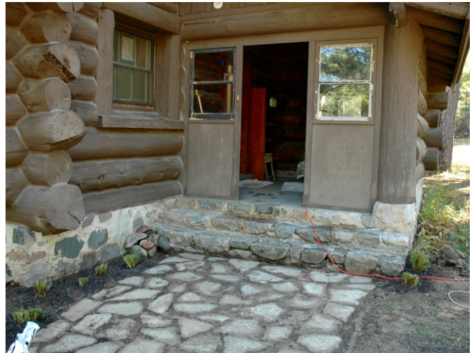
Stone walkway uncovered at Discovery Center back door. It was placed there by the first forester to live in the building, Bill Horsell, circa 1936.
