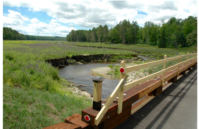
The silt bed is covered now with natural vegetation. The timber bridge has new railings to increase safety during winter snow cover.
