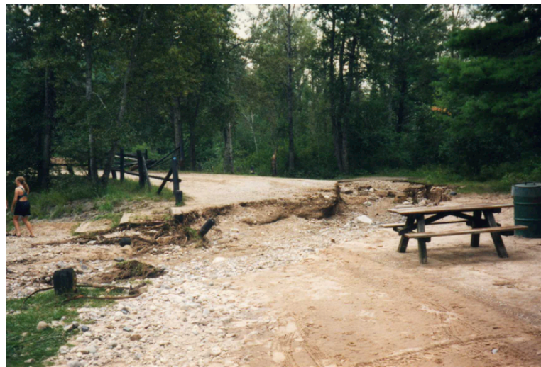
A storm in 1995 overflowed the culverts and washed out Ford Lake Road that spans the Pigeon near Pigeon River Campground. A campsite on the right beyond the picnic table will become a parking area when the culverts are replaced by a timber bridge.
