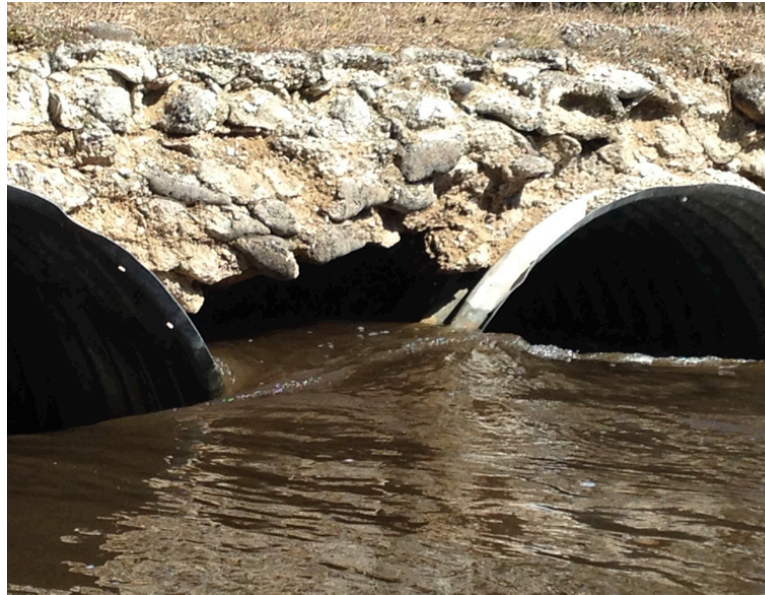
Embankment surrounding culverts is eroding.
